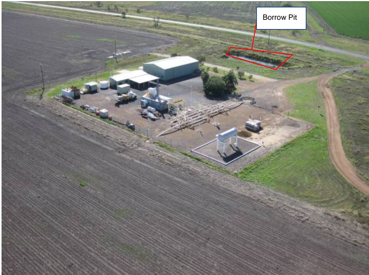
Plate 3: Existing Dalby Compressor Station
