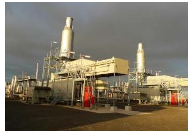
Wollert compressor station, Vic
