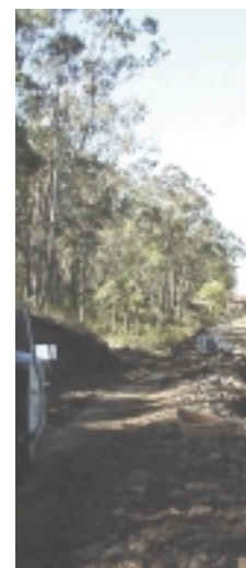
Roma to Brisbane Pipeline System Looping stage five (Wallumbilla to Ipswich) during construction (RBP Looping).
